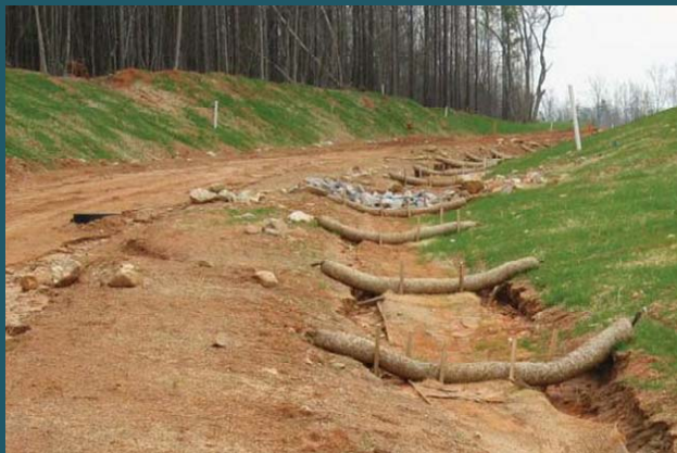
Check dams are constructed of rock or other materials across a drainage ditch to mitigate erosion by reducing water flow velocity.
