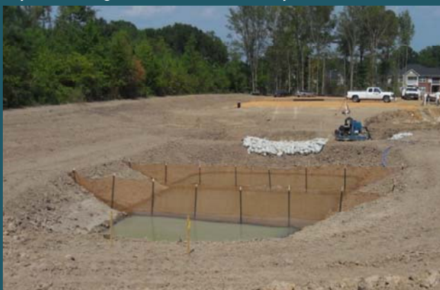
Sediment basins are low earthen dams across drainage ways that create a temporary storage pool.
