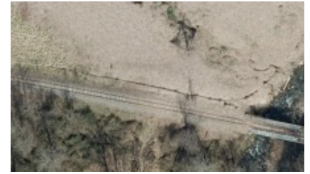
North Pacolet River Heavy Erosion (35.220, -82.326) Heavy erosion along the north side of the rail line and along the shore of the North Pacolet River.
