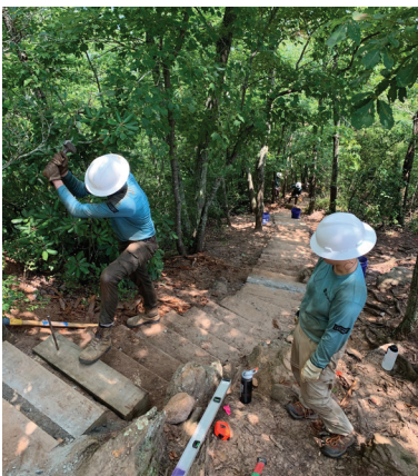
CCNC repairing steps on the Backside Trail at Crowders Mountain State Park
