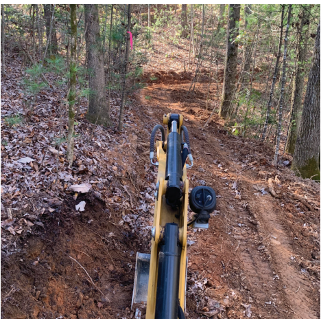
Putting training to use with mini-excavator at Lake James State Park with CCNC crews
