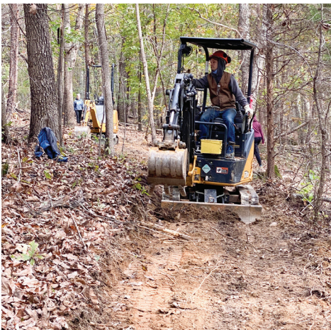
Piedmont Region Trail Specialist using mini-excavator to finish grading trail cut by trail dozer at Crowders Mountain State Park
