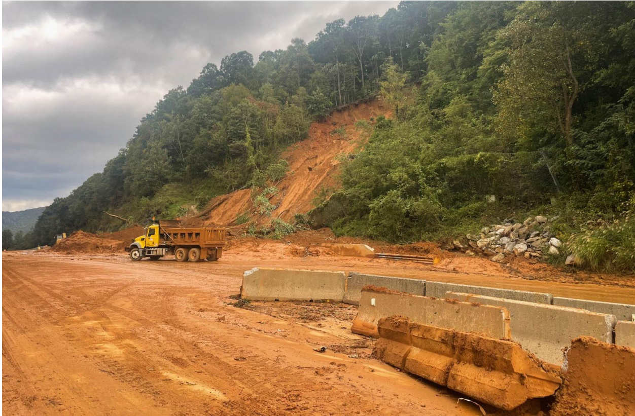
Figure 10: Aftermath of Helene-Triggered Mudslide, September 28, 2024 (Credit: NCDOT)
