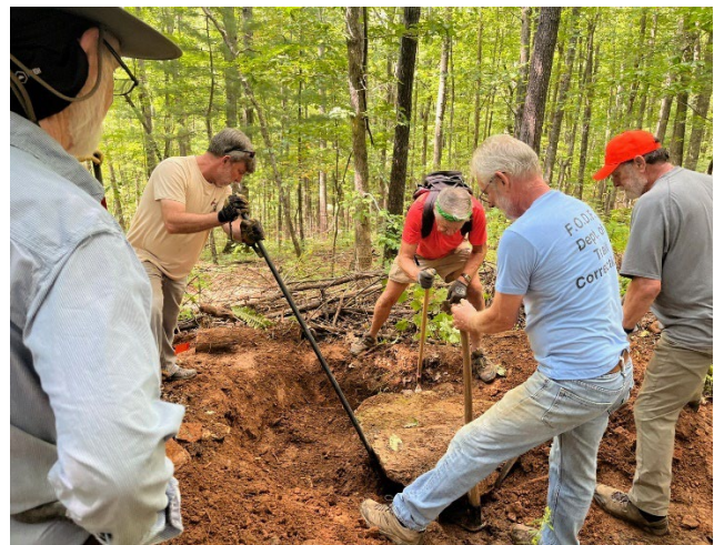
Friends of DuPont Forest volunteers maneuvering a large rock as part of a trail repair and restoration project.
