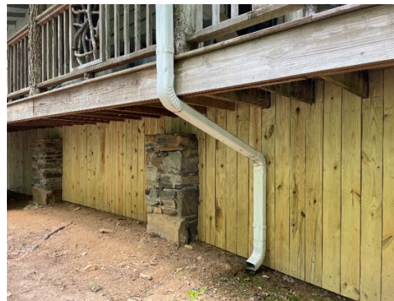
A section of the completed lower level enclosure of the law enforcement cabin.
