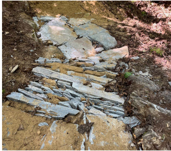
Rock armoring installed along Jim Branch trail to repair severely degraded section of trail.
