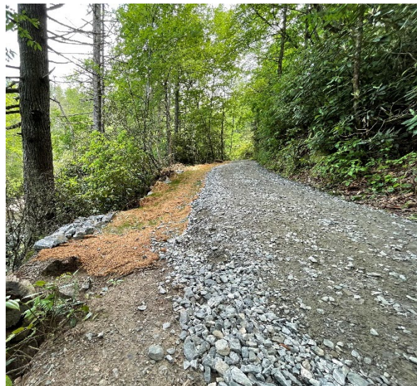
Triple Falls Trail added an improved walking surface and erosion control measures.
