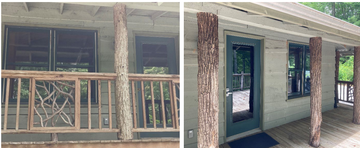
New glass in the exterior doors and new windows at the law enforcement office.
